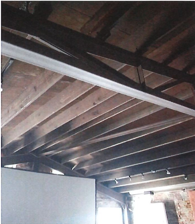
Second Floor Steel trusses and 2x 16 wood rafters as a "Memory" or historic reference of the former wood framed roof support system
