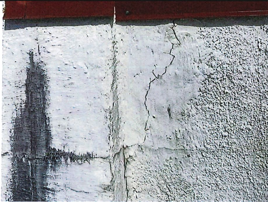
Cracks in facade with algae damage.
