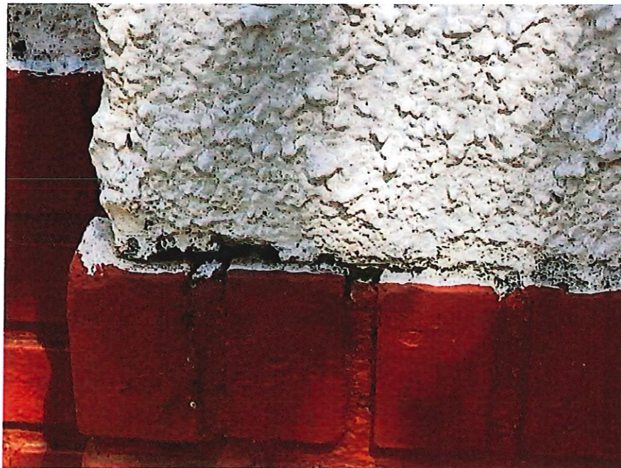
Stress crack above stucco to brick transition.
