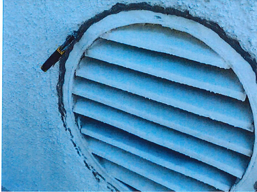
Sealant failure around louver vent.
