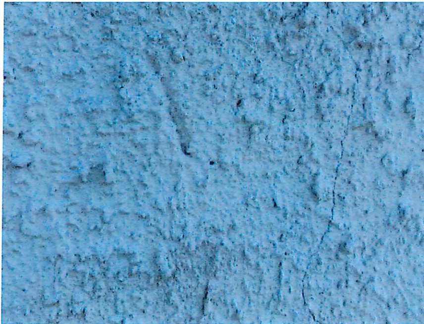
Pinholes in facade.
