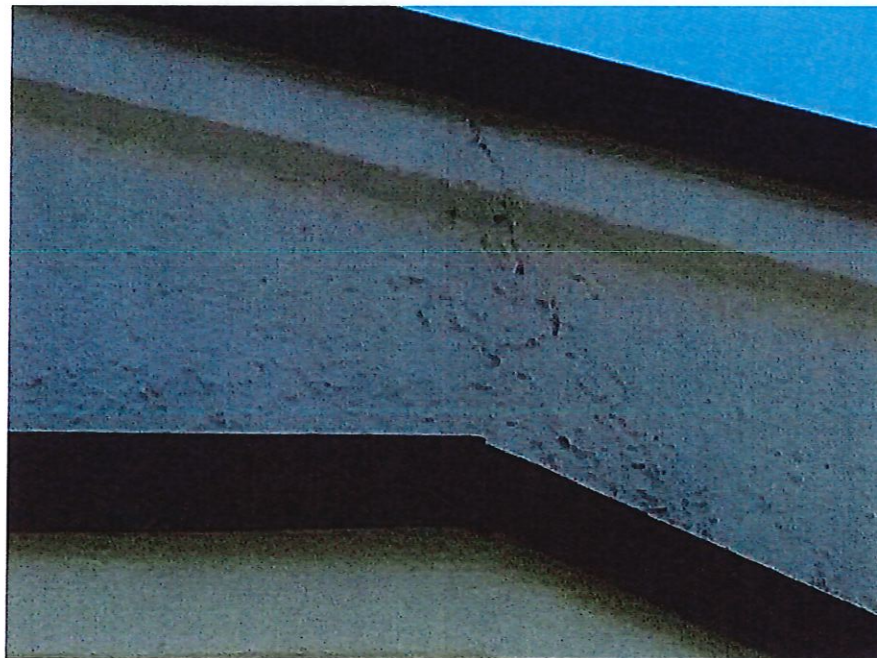
Stress cracks in facade.
