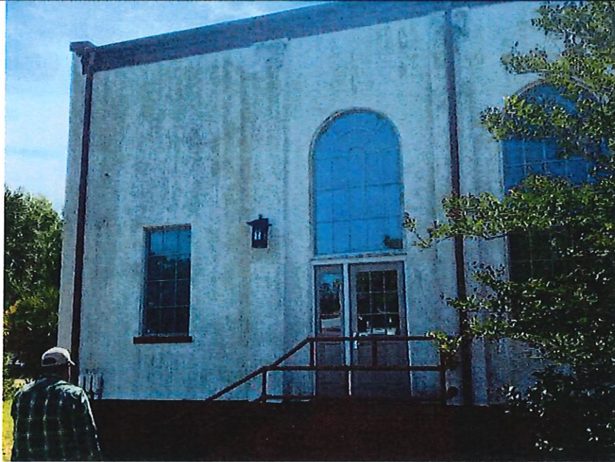
Algae damage on facade.
