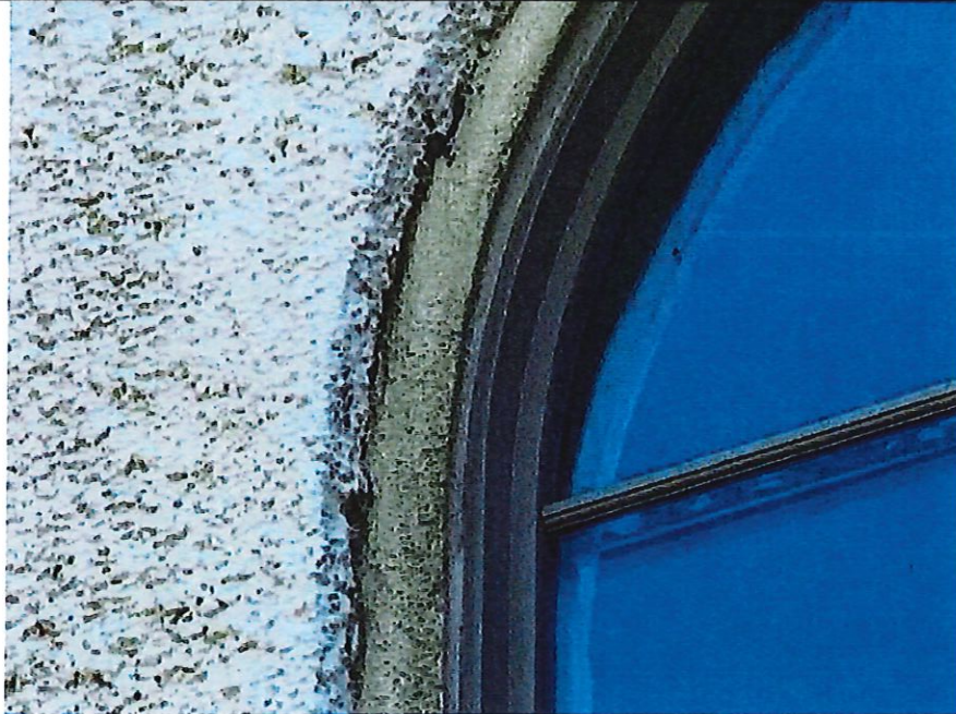
Sealant failure around window.
