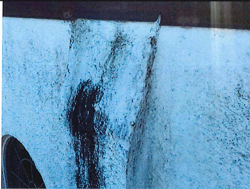
Algae damage on facade.
