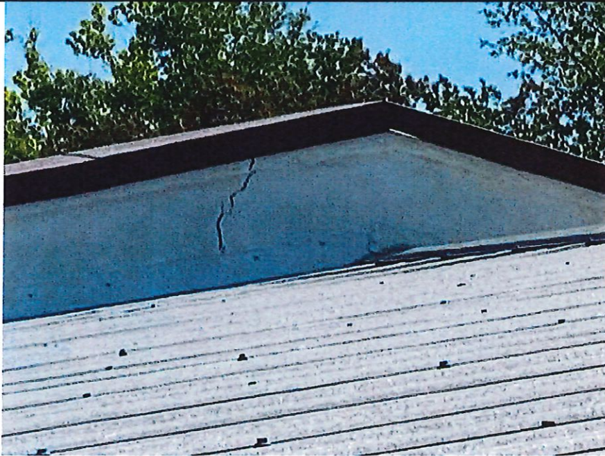
Stress crack in facade.
