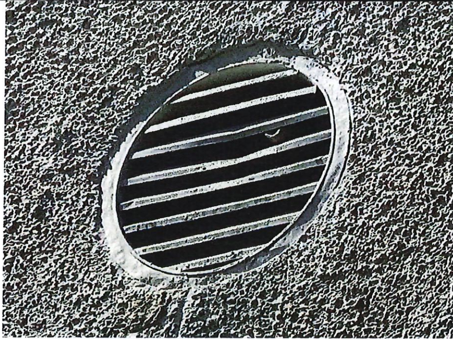
Sealant failure around louver vent.
