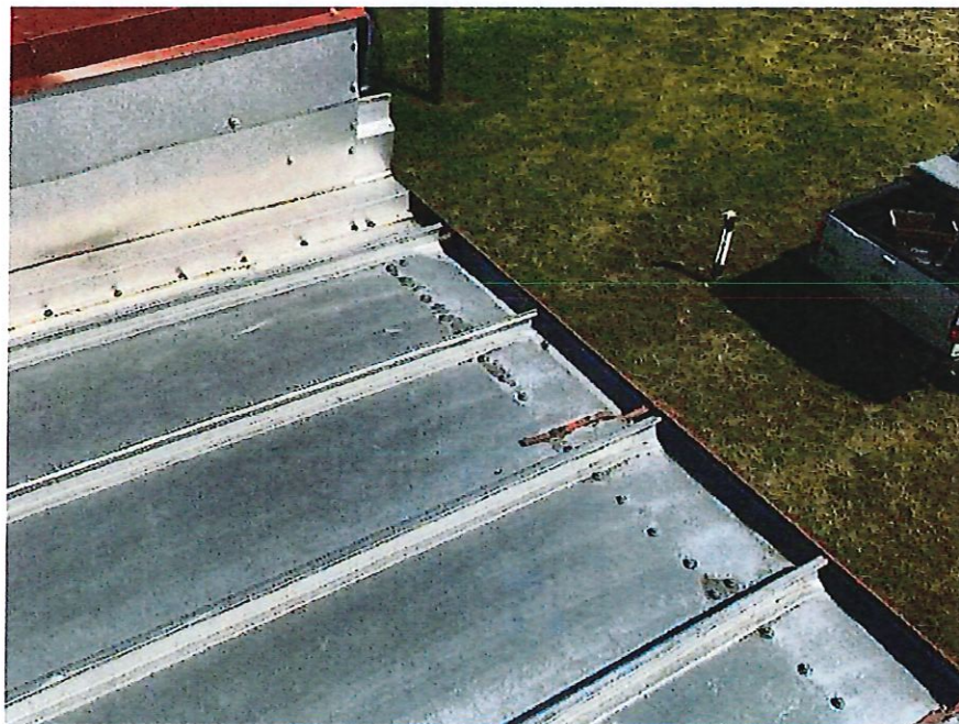
Early oxidization on gutter straps.
