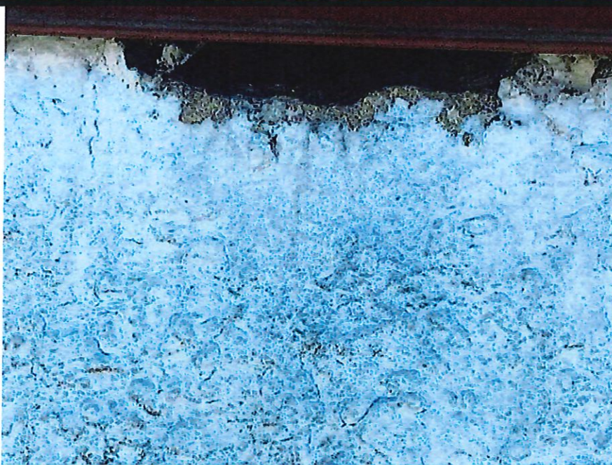
Facade deterioration allowing water intrusion.
