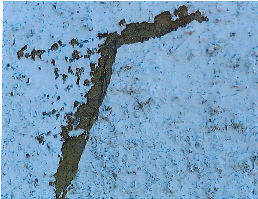
Crack in facade allowing water intrusion.
