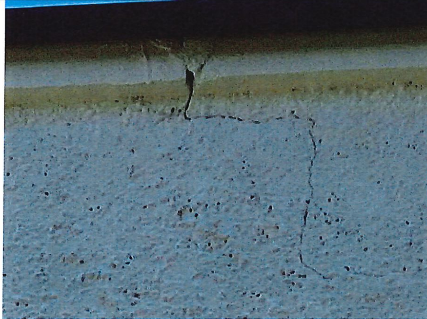
Stress cracks in facade.
