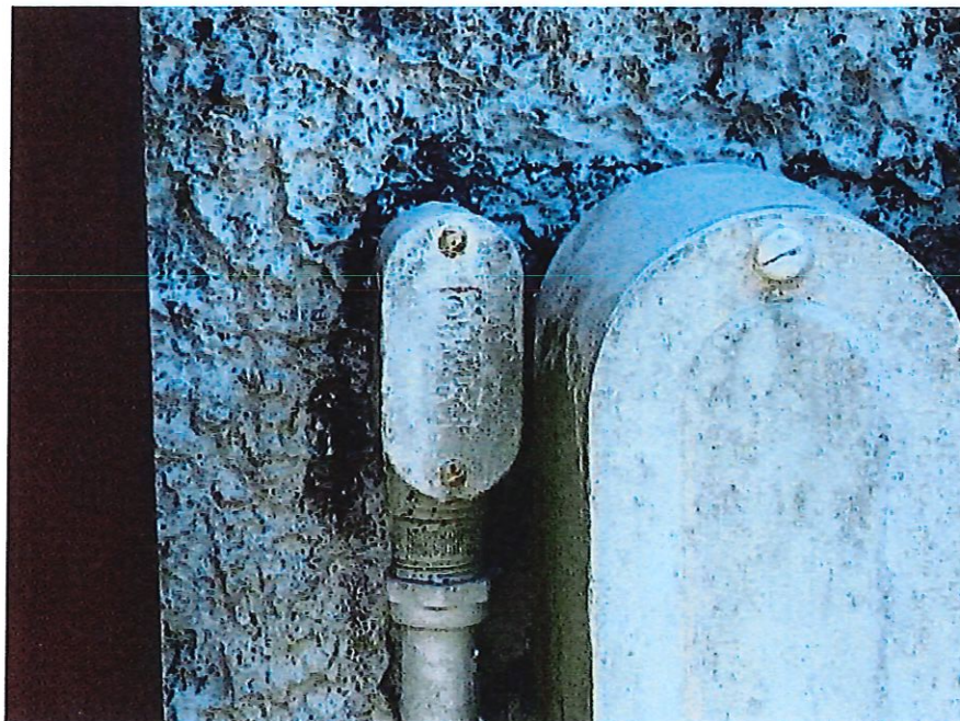
Opening around conduit lines.
