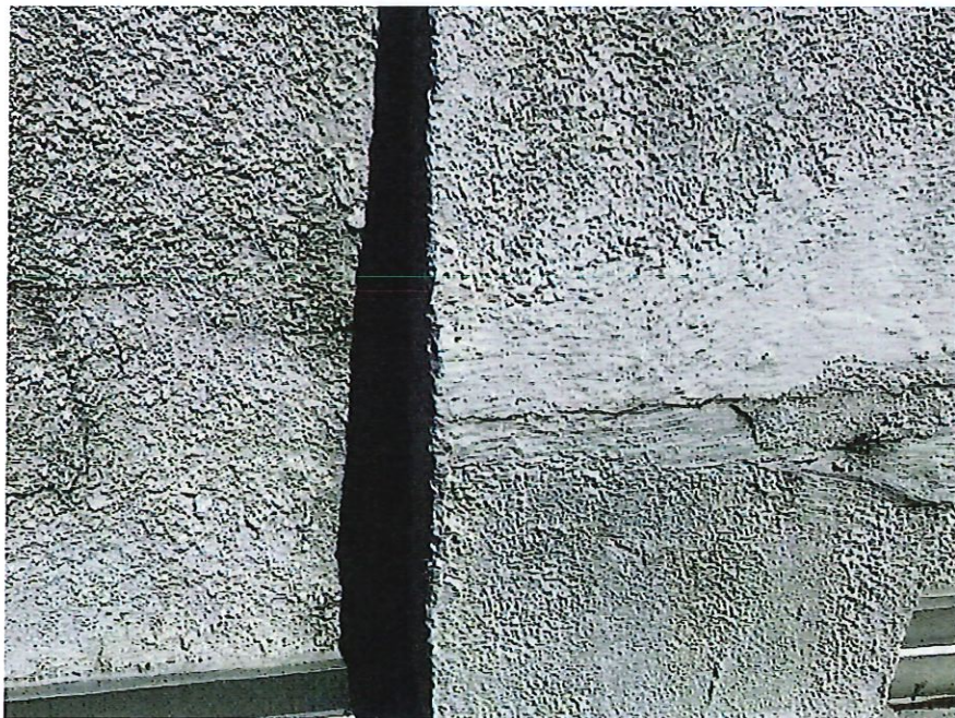
Cracks in facade.
