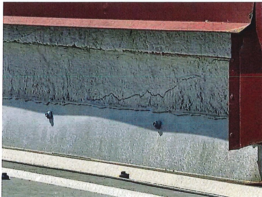
Stress cracks in facade.
