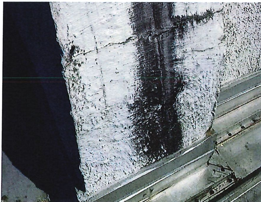
Cracks in facade with algae damage.
