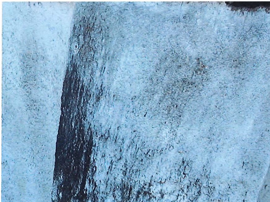
Algae damage on facade.
