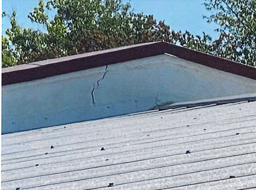
Stress crack in facade.
