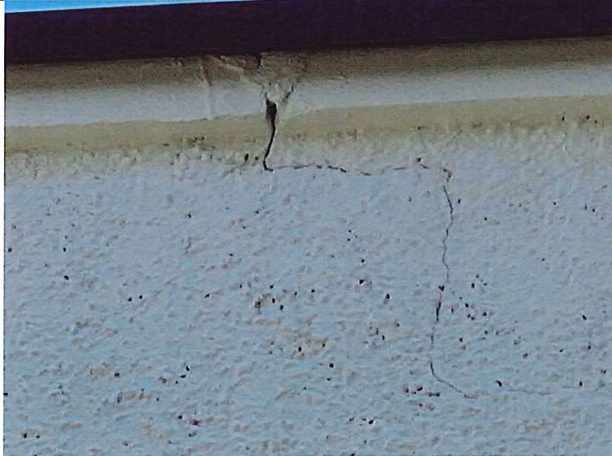
Stress cracks in facade.
