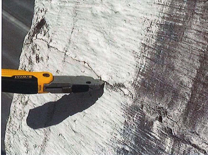
Cracks in facade allowing water intrusion.
