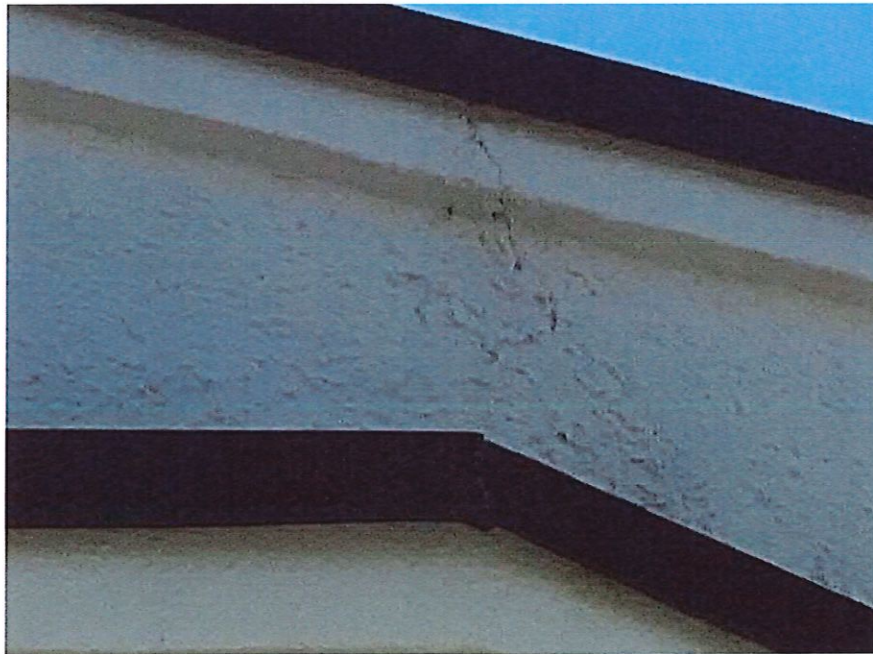
Stress cracks in facade.
