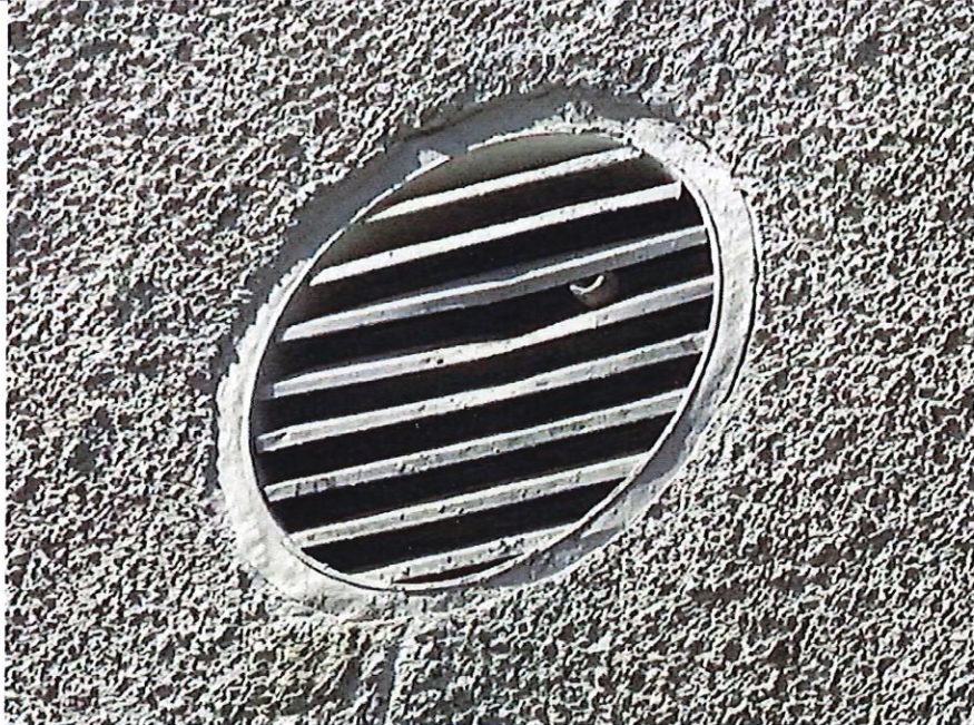
Sealant failure around louver vent.
