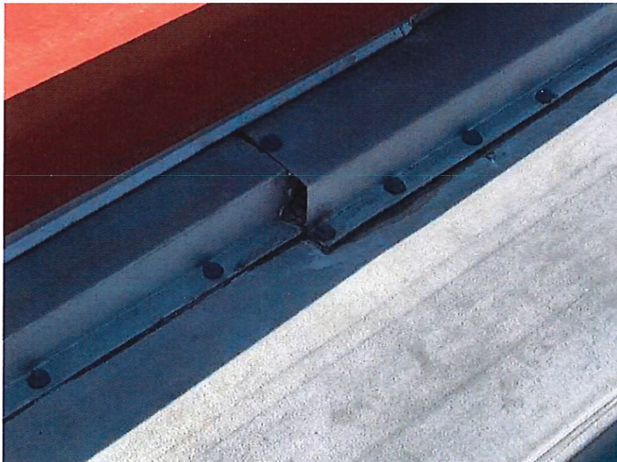
Opening at rake edge allowing water intrusion.
