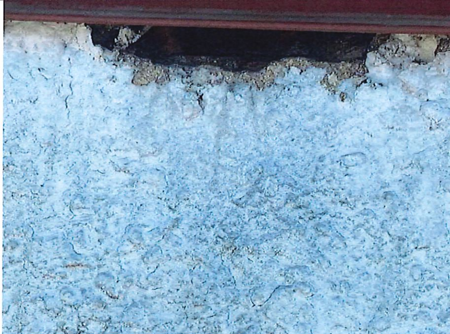
Facade deterioration allowing water intrusion.
