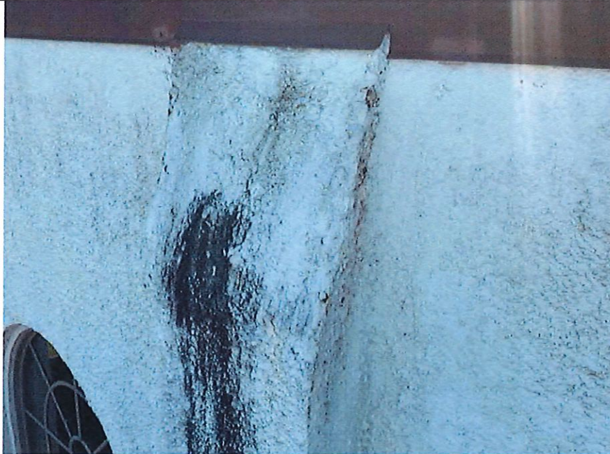
Algae damage on facade.
