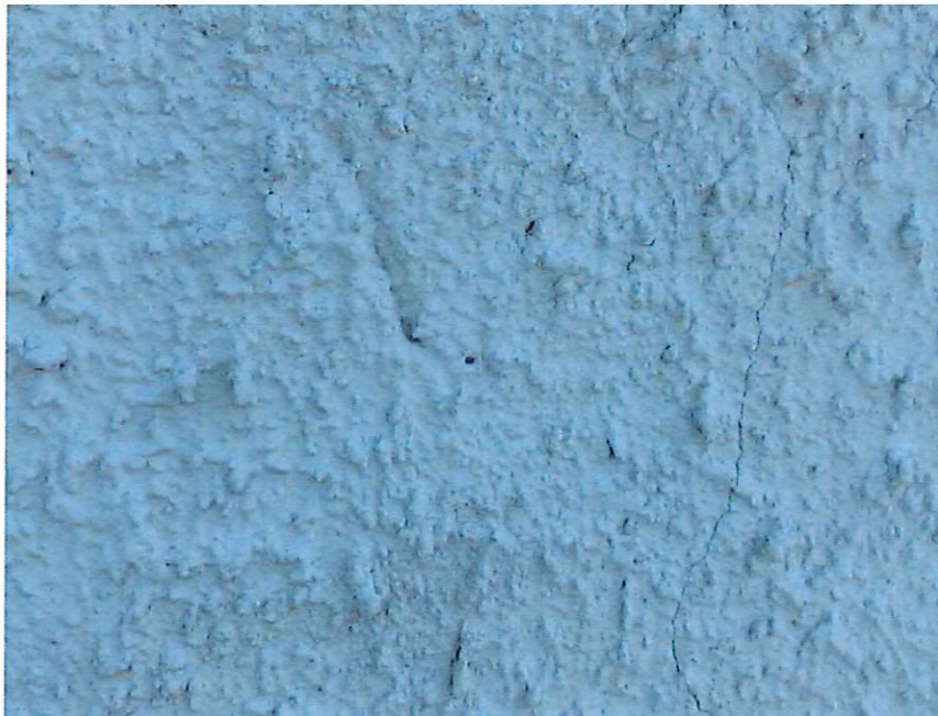
Pinholes in facade.
