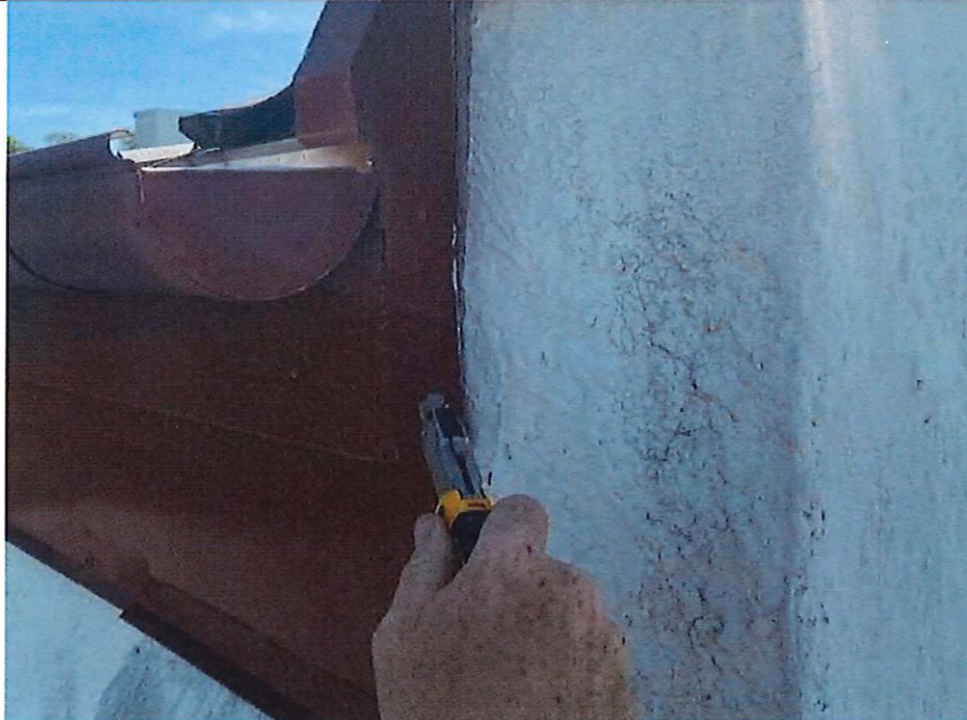
Sealant failure around eave.
