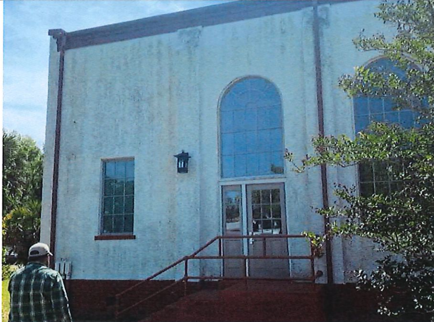
Algae damage on facade.
