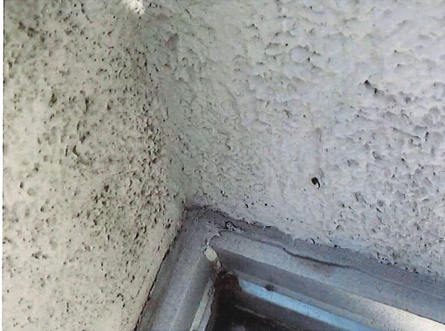
Sealant failure at counter flashing.
