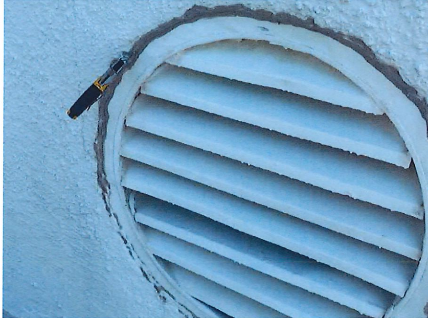
Sealant failure around louver vent.
