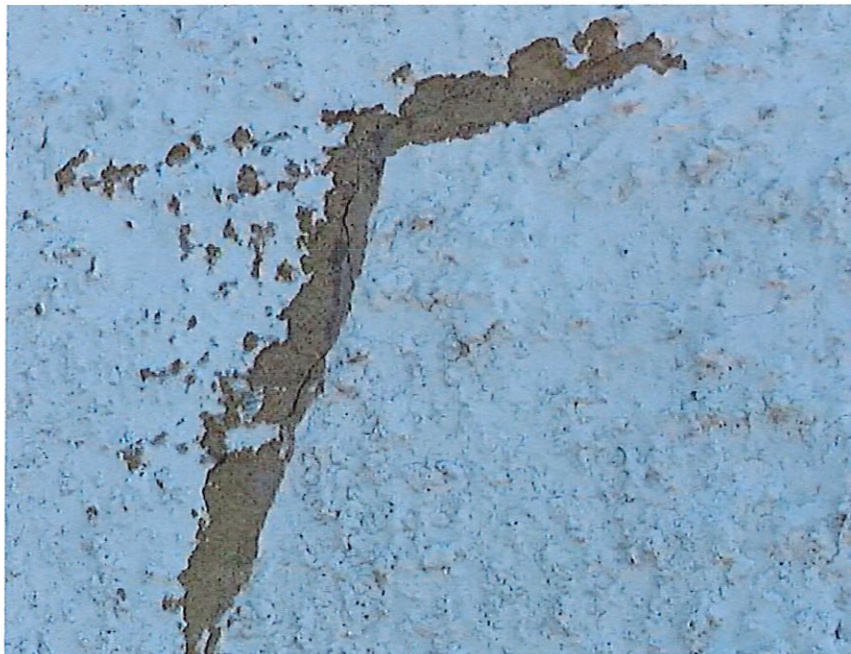
Crack in facade allowing water intrusion.
