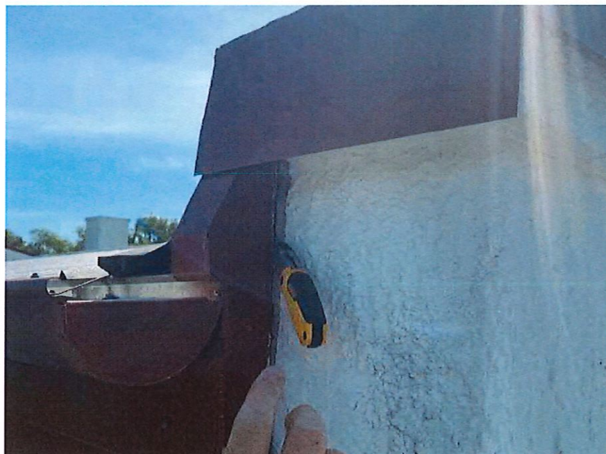
Sealant failure around eave.
