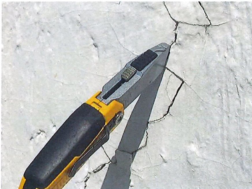
Cracks in facade allowing water intrusion.
