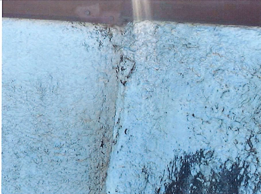
Stress cracks on facade.
