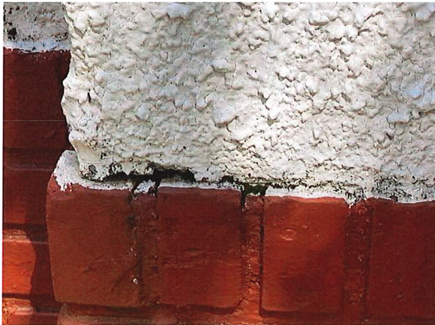
Stress crack above stucco to brick transition.
