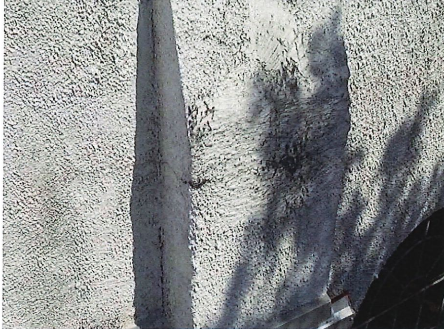
Cracks in facade.
