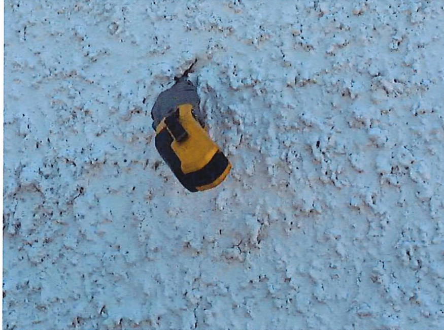
Crack in facade allowing water intrusion.
