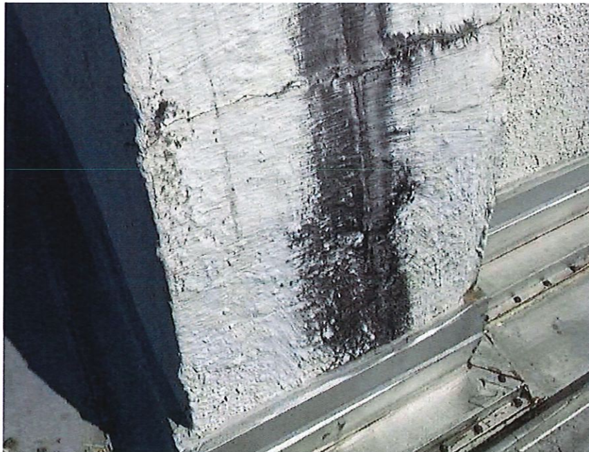
Cracks in facade with algae damage.
