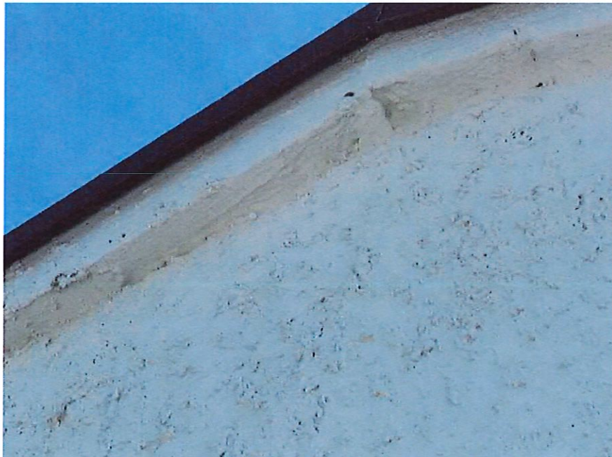
Rake edge not completely sealed.
