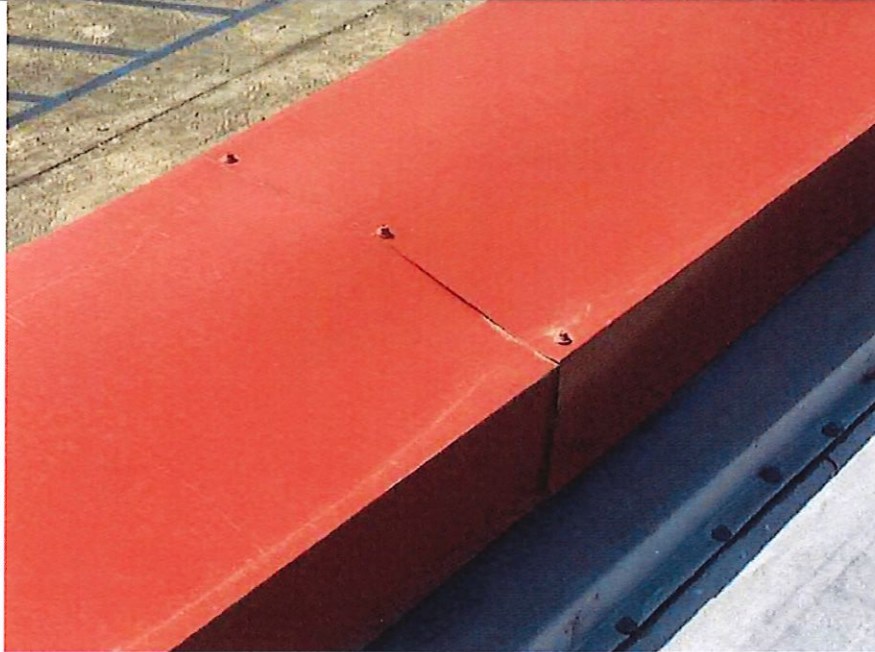
Butyl tape failure on coping joint.
