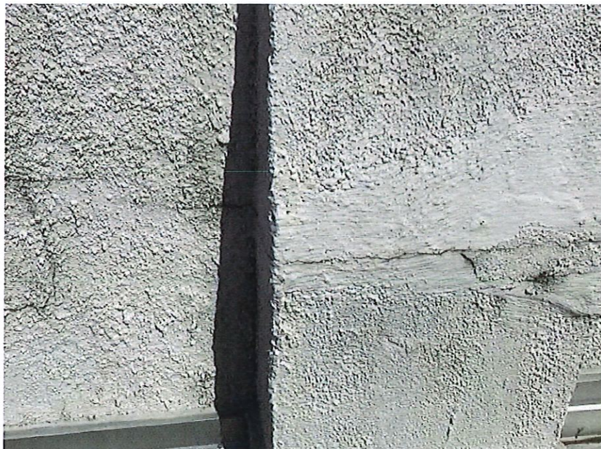
Cracks in facade.
