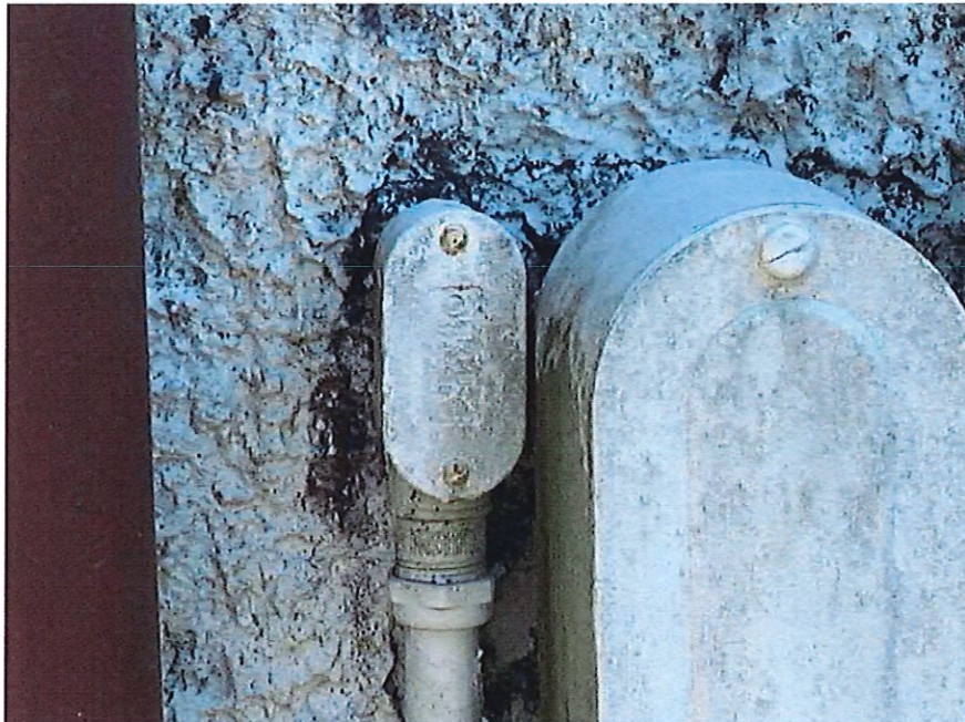
Opening around conduit lines.
