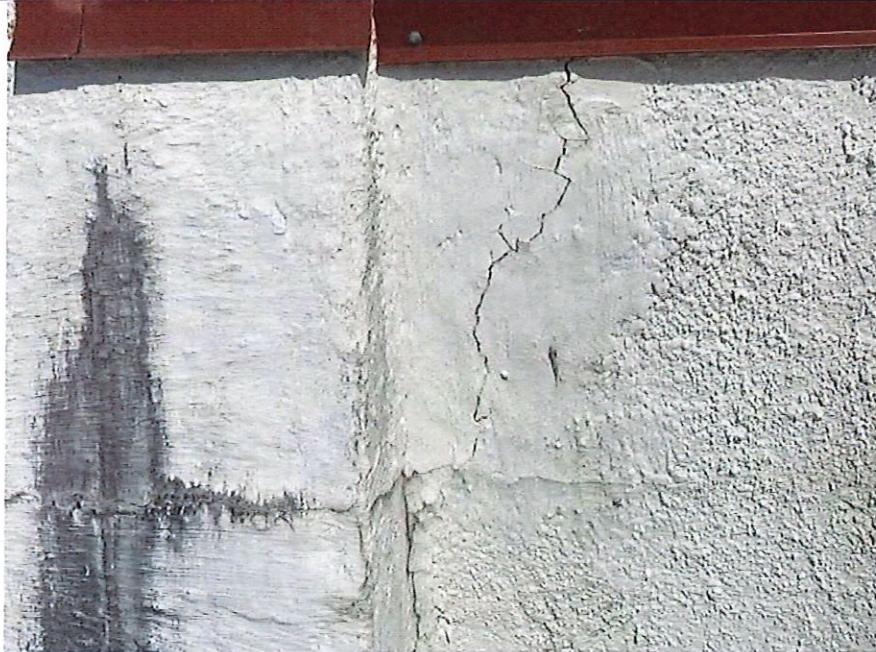
Cracks in facade with algae damage.
