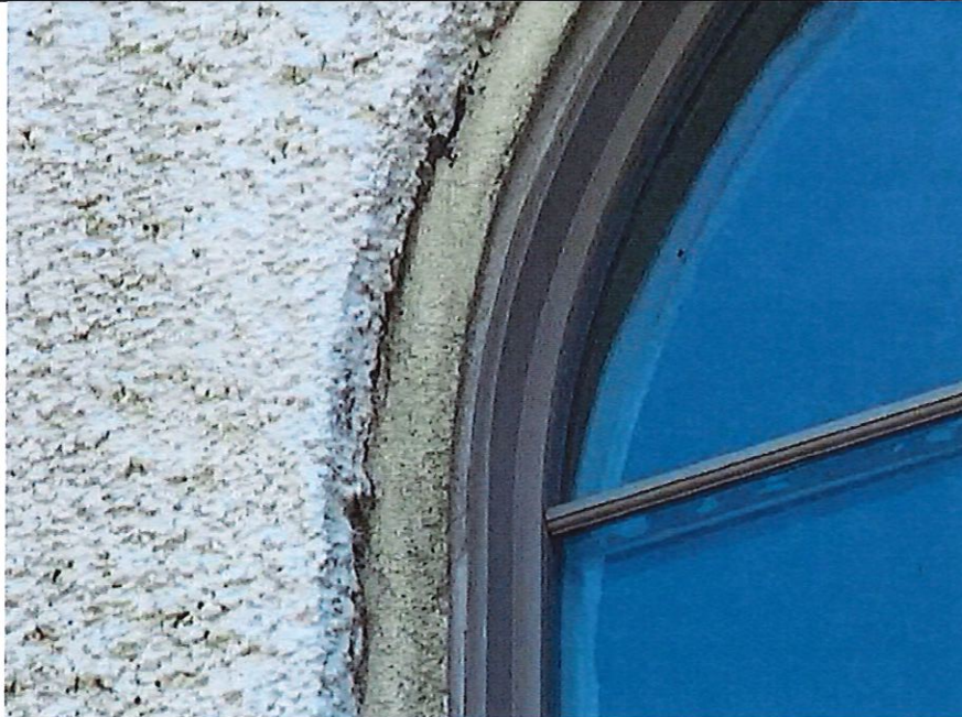
Sealant failure around window.
