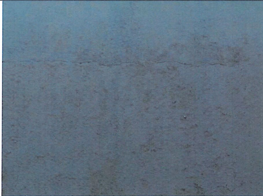
Stress cracks in facade.
