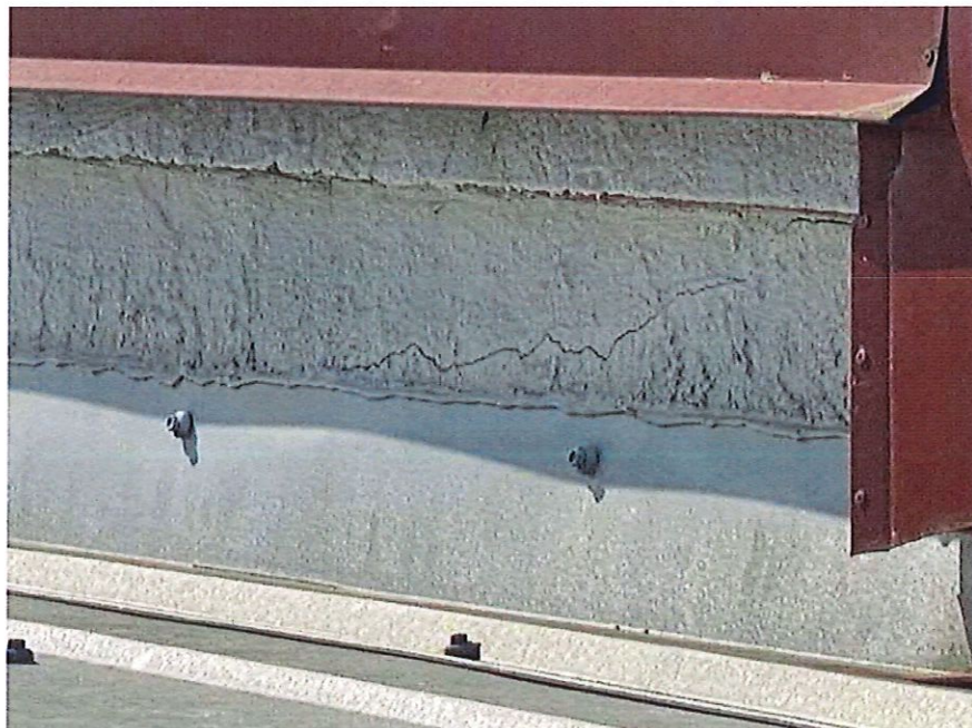
Stress cracks in facade.
