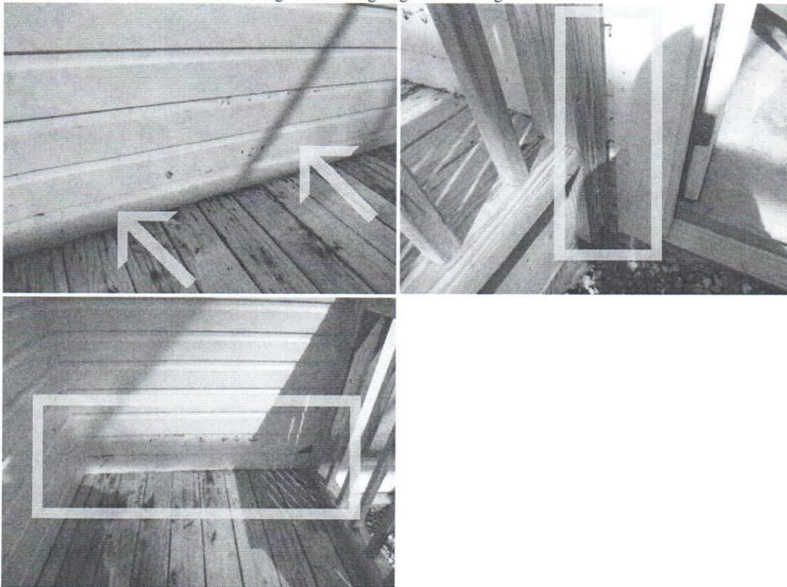
20. Wood rot noted on exterior siding: rear deck area siding right of the garage patio door.
