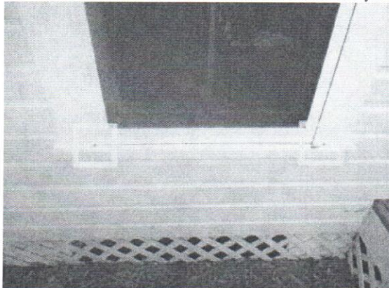
44. Wood rot noted on the exterior trim: left side yard master bedroom window trims.
