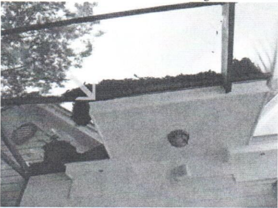
37. Wood rot noted on the exterior trim: rear hall bedroom patio door frame.
