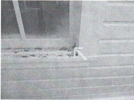
41. Wood rot noted on the exterior trim: left living room window.
