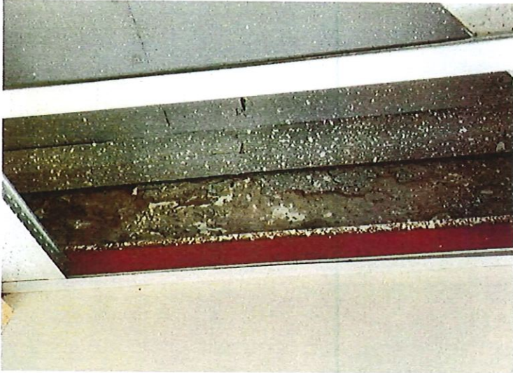
Previous steel supporting frame in Middlebrook Building. Note Fireproofing in the form of double layers of gypsum Board required by building code, located below historic wood timber frame. The added weight of these elements contribute to the sagging floor frame condition.
