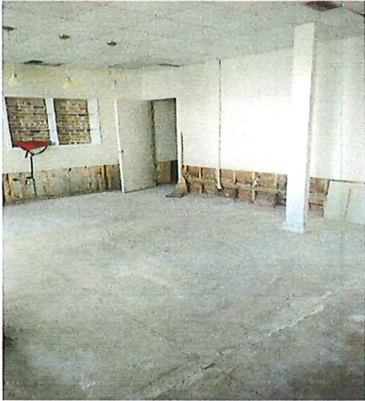
Photo shows depth of false perimeter wall supporting 2nd floor structure. Note lower 27" of gypsum and insulation has been removed due to flood damage
