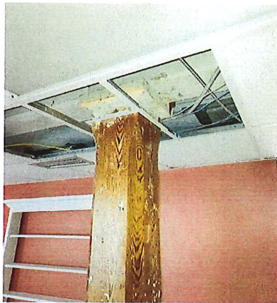
Original wood column at mid span Note original wood beam supporting Second floor frame
