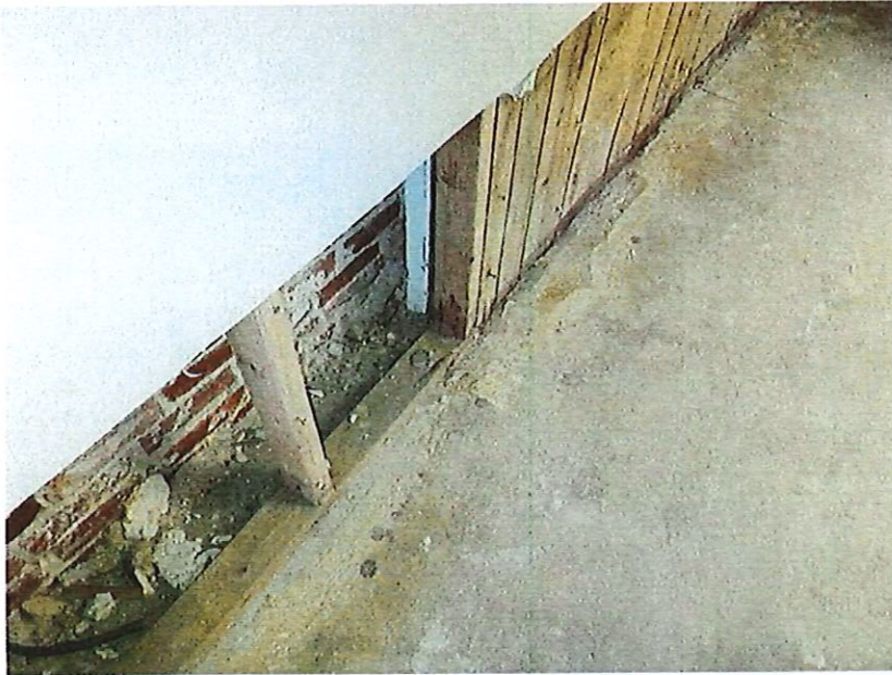
Common Wood Stud with gypsum drywall finish cut back due to flooding from Hurricane Michael' 10-10-2018. Note: Saturated insulation has been removed. Mold spores are present at floor level and wood rot is indicated at the wall sill plates despite being built with pressure treated wood material.
