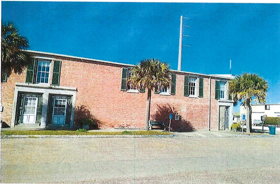
1 st floor windows require replacing. 2nd floor windows to be refinished
