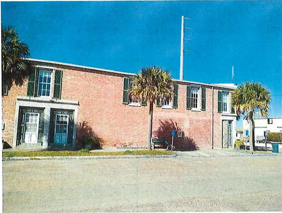
East Elevation of Middlebrook Cotton Warehouse/Exchange – 1 Avenue "E" Note granite lintels and columns at fenestration. It appears a series of lintels and openings have been removed near the north end of the building.
